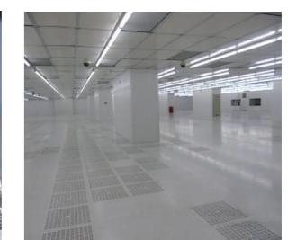
Biel Crystal, Hongkong Aluminum raised floor(conductive vinyl), 6,400m 2
